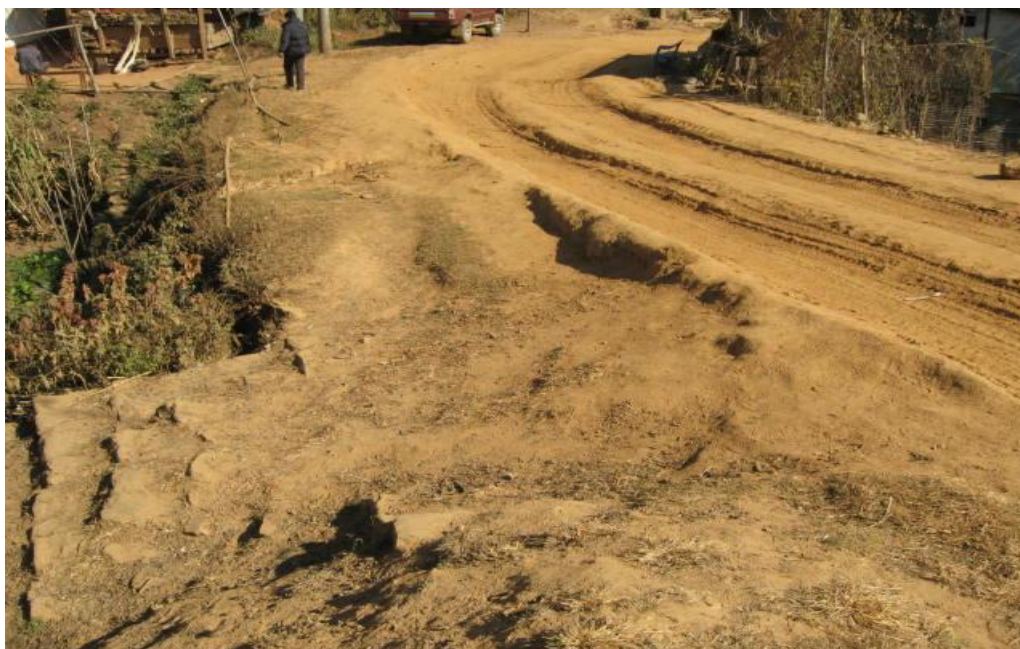
Figure 3.4 Deep Undulation Created in Poorly Maintained Road in Nepal
