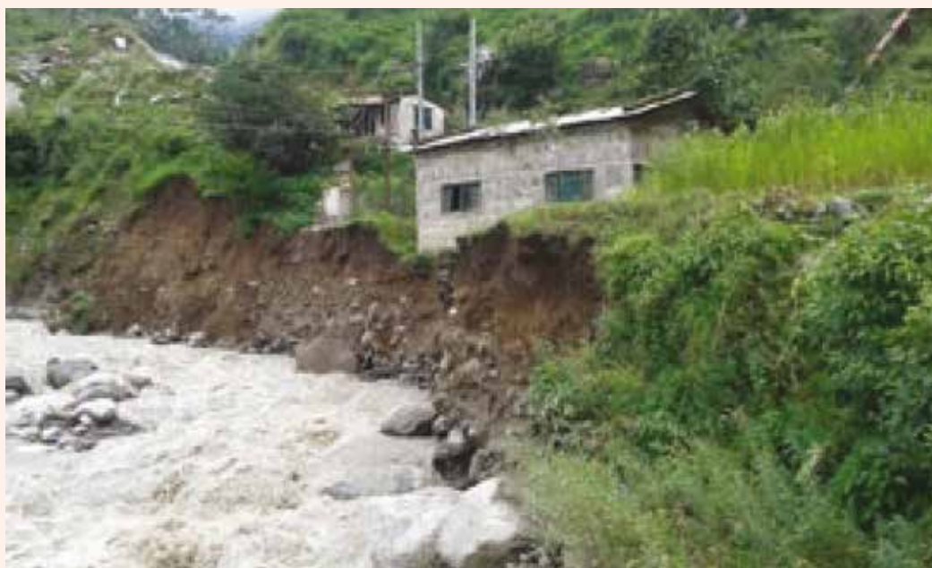
Figure 4 Power house of the Triveni Micro Hydropower Project at risk by the Bahuli Rivulet, in Martadi of Bajura (Source: Prakash Singh) http://www.the-himalayantimes.com/fullNews.php?headline=Bajura+headquarters+in+dark+for+five+days&NewsID=424456#sthash.77OQPrqW.dpuf
