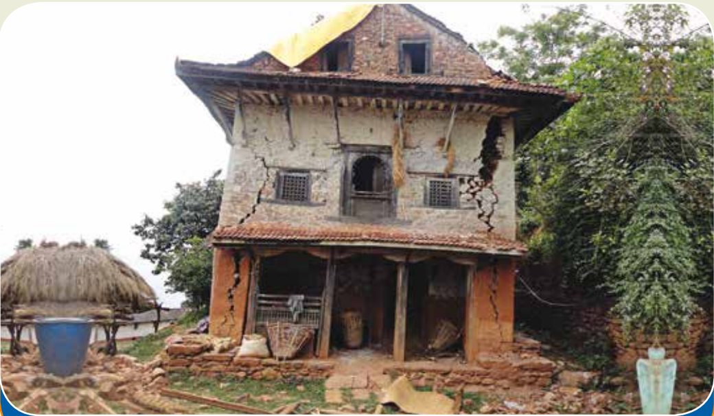
A Rural House Damaged by Gorkha Earthquake
