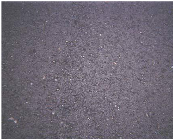
Figure 4: Unsuitable Surface, Dense Graded HMA With Closed Surface
