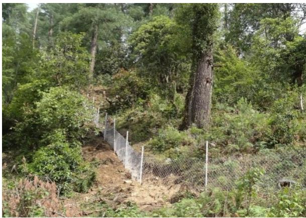
Fig. 8: Mess wire fencing to control wildlife
