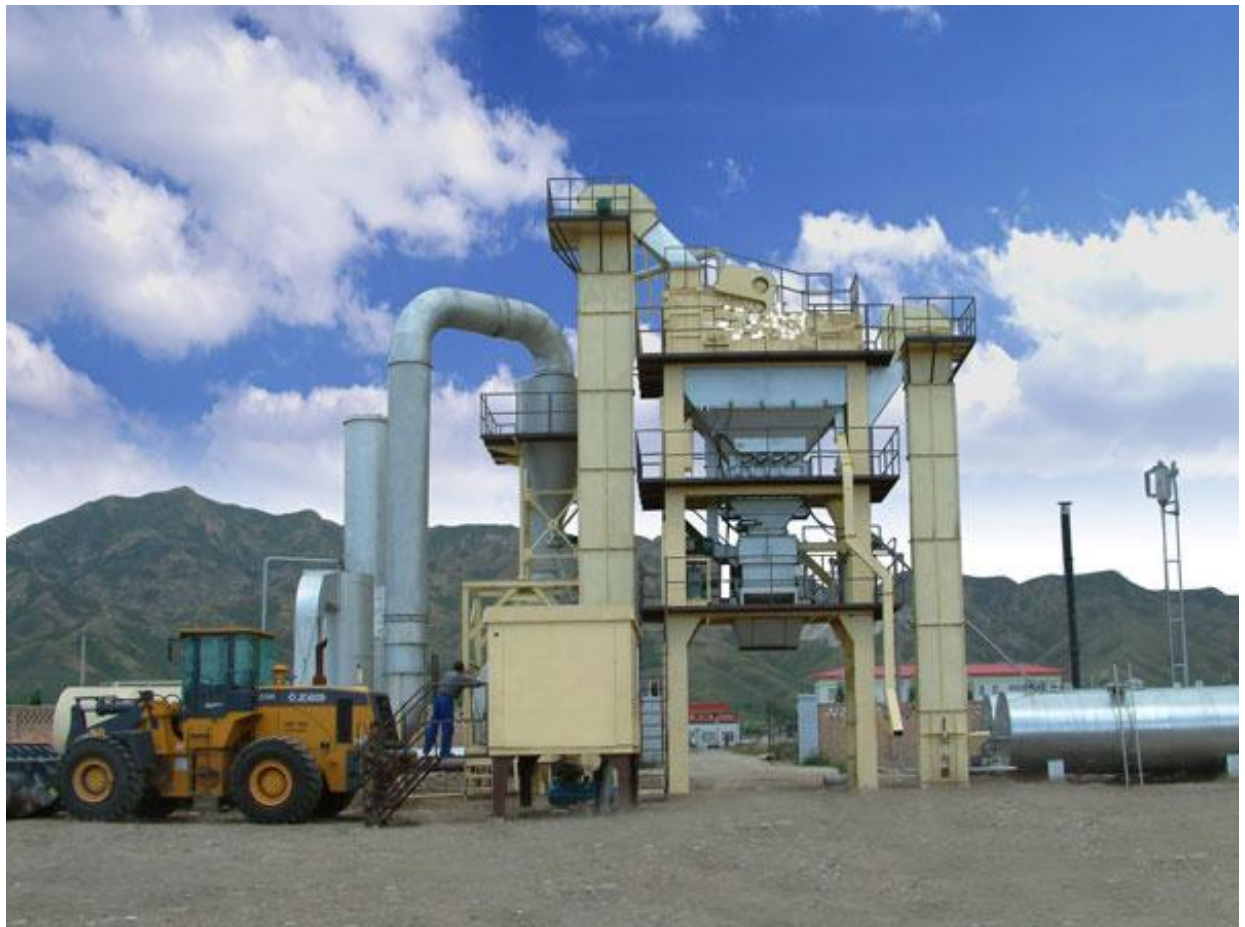
Figure 4.1 Typical Batch Plant
