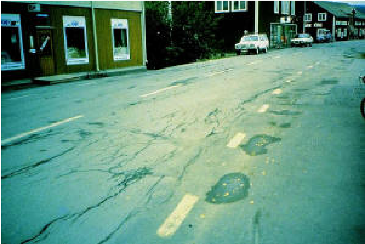
Figure 9.1. Frost heave on a city street in central Sweden.
