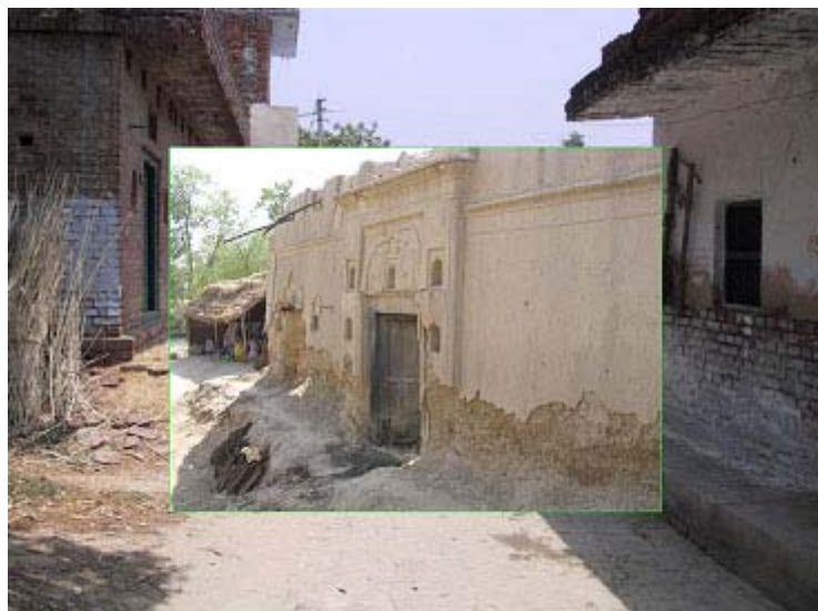
Settlement at risk in waterlogged areas of canal command
