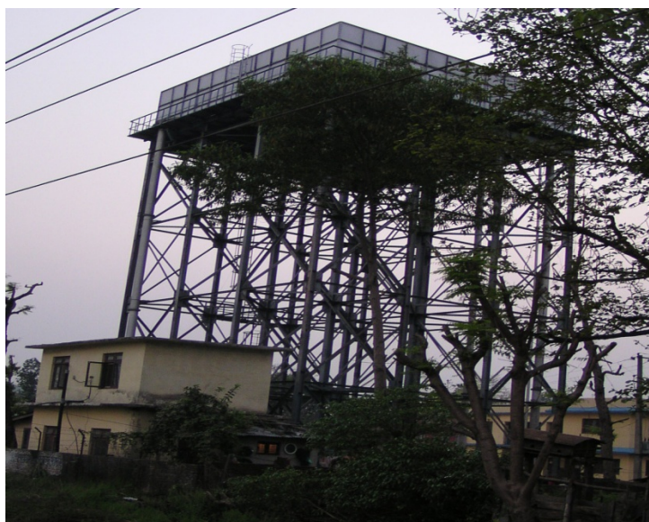
Figure 11: Water Supply Overhead Tank, Bharatpur
