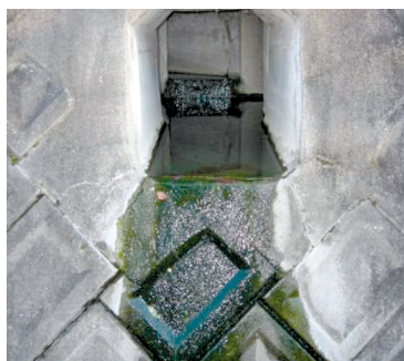
Figure 7.1b: Gutter with Discharged Treated Effluent from a Johkasou
