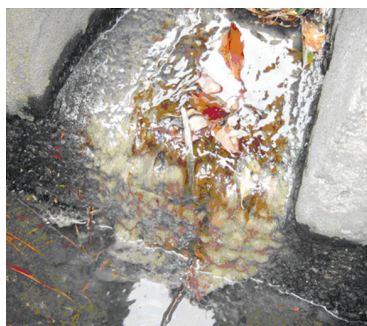
Figure 7.1a: Gutter with Untreated Gray Water Discharged in a Tandoku-shori Johkasou Area
