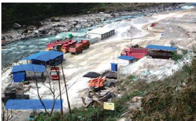
Aggregate Crushing Plant
