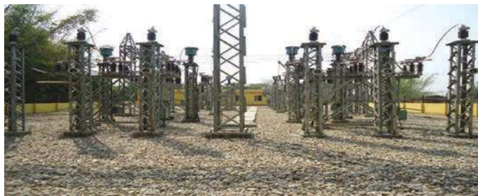
Completed Dhulabari 33/11 kV, 6/8 MVA Substation
