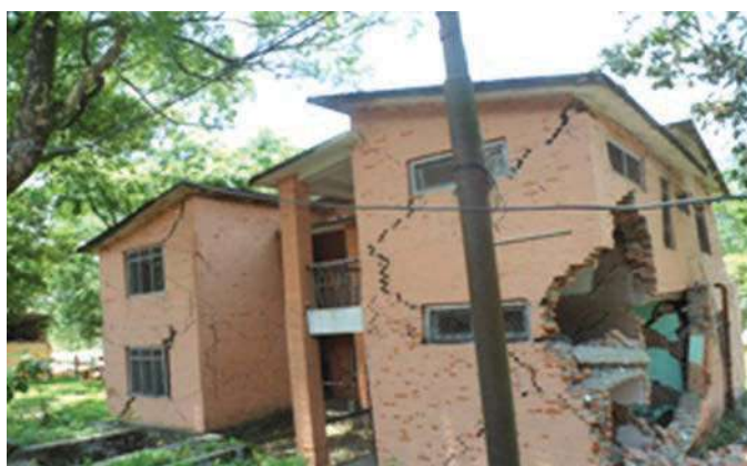
Ravaged Masonry Building
