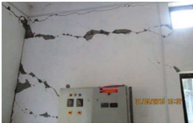
Damaged inside wall
