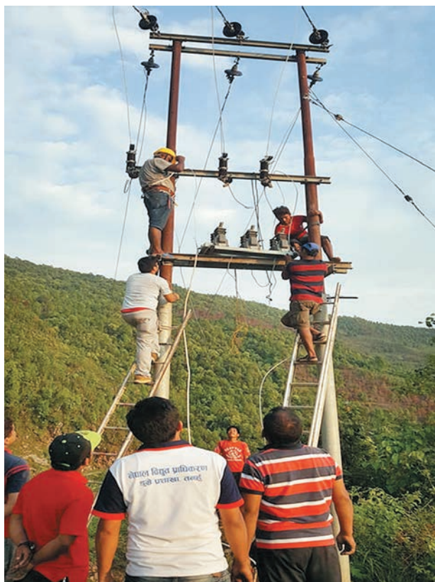
HT Metering Installation at Dharampani Cummunity
