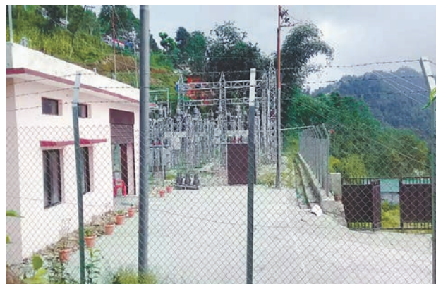
33/11kV Okhaldhunga Substation, Gorumare Bhanjyang, Okhaldhunga (now in operation)
