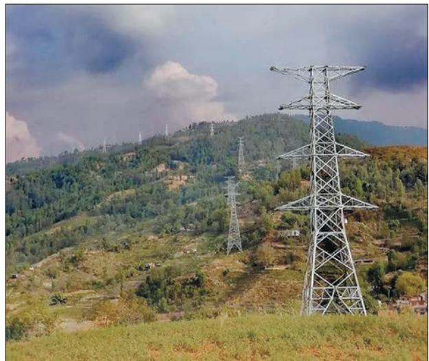
220 kV Transmission Tower
