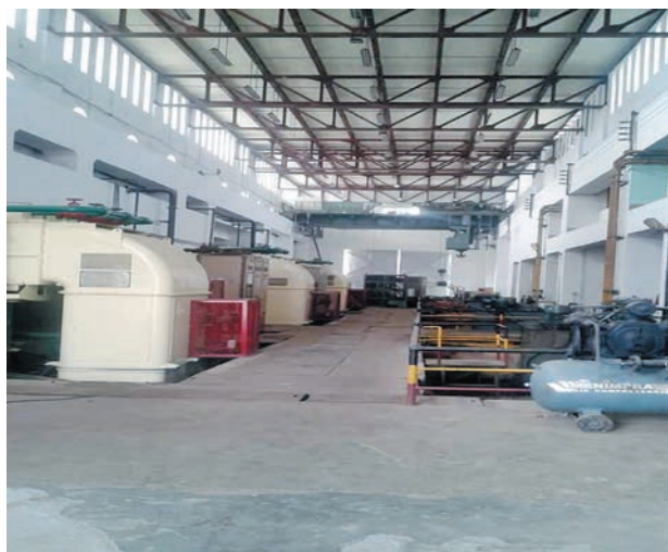
Gandak Power House
