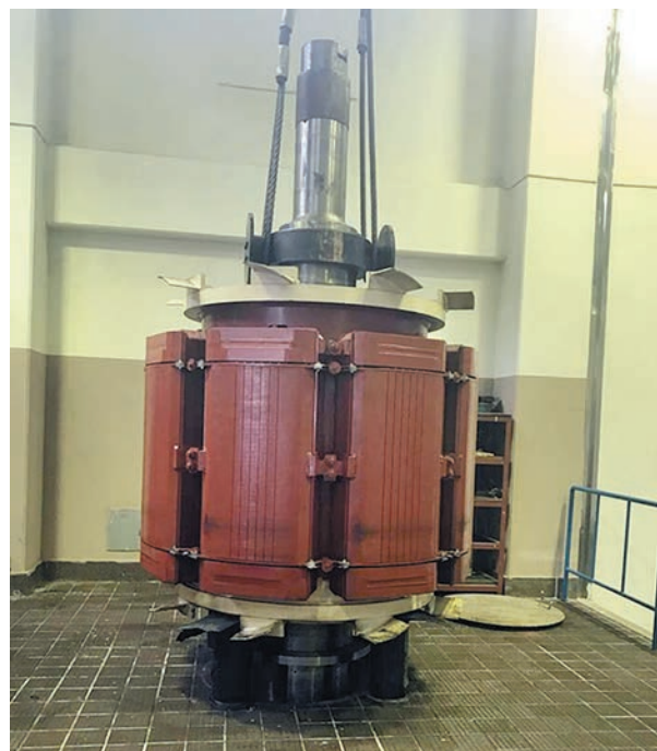
Rotor Assembly of Unit No. 2
