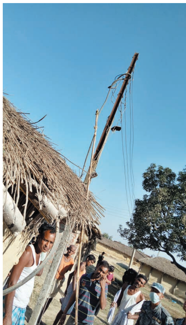
Three phase meter hooking arrangement found
