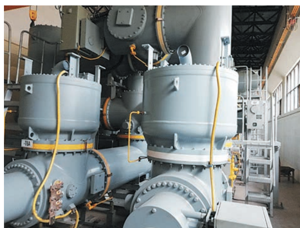
Newly Installed GIS Potential Transformer
