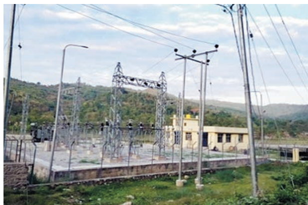
Construction Power Sub-station of Tanahu HEP.
