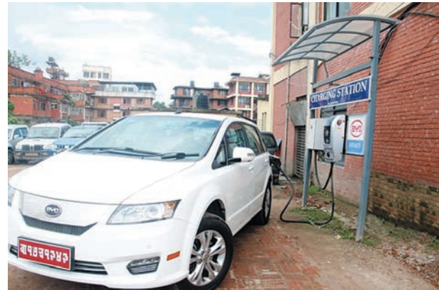
Electrical Vehicle Charging Station at Ratnapark Distribution Centre
