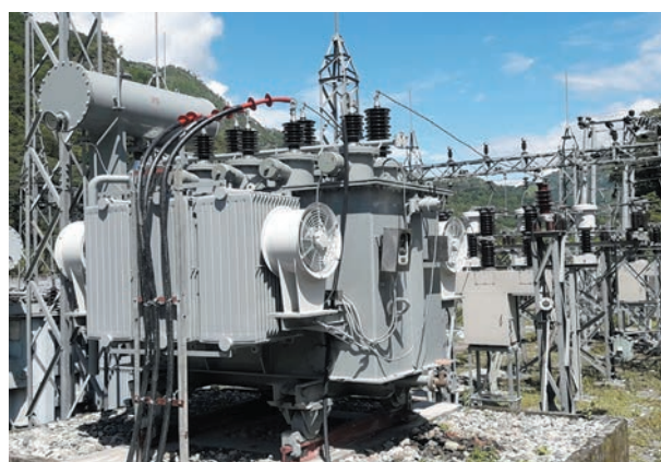
33/11 KV, 6/8 MVA Power Transformer Upgrade at Myagdi Substation
