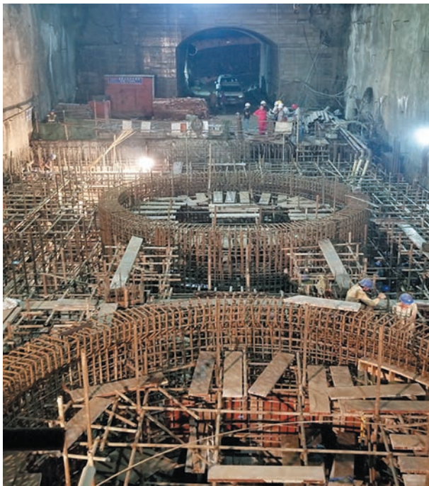
Underground Power House
