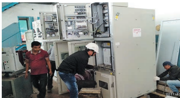
Commissioning of Unit-2 GCB with Protection Relay
