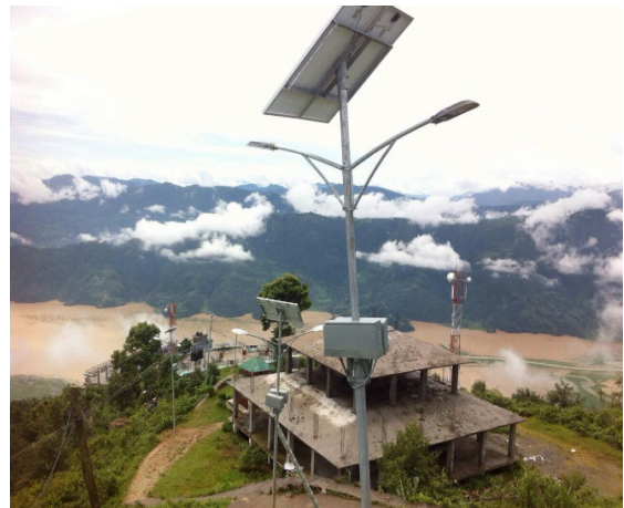
Installed solar power lights at Sarangkot
