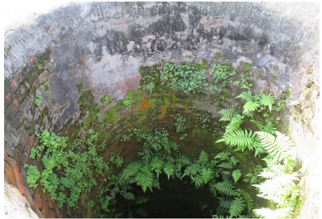
Well before maintenance
