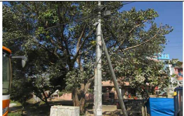
Figure 11. Electric pole no. 14
