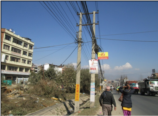
Figure 30. Electric pole no. 20
