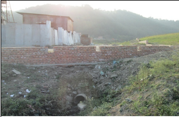
Figure 18. Surface sewer and storm water drain mid point
