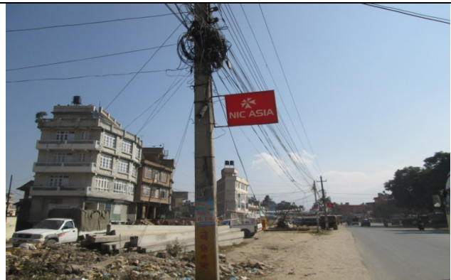
Figure 62. Electric pole no. 39
