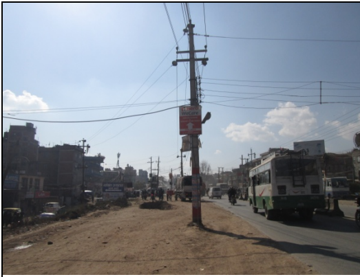
Figure 66. Electric pole no. 52
