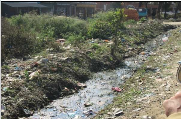
Figure 52. Surface storm water drain
