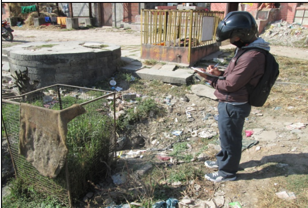
Figure 7. Storm water drain inlet
