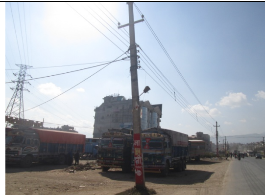
Figure 57. Electric pole no. 43
