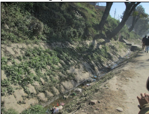
Figure 127. Surface storm water drain
