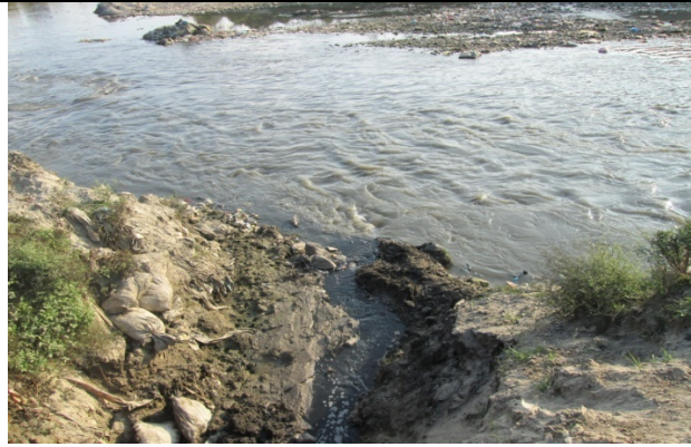
Figure 19. Surface sewer and storm water drain Outlet
