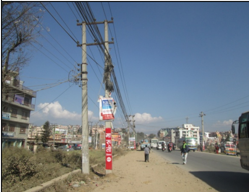
Figure 40. Electric poles no. 25
