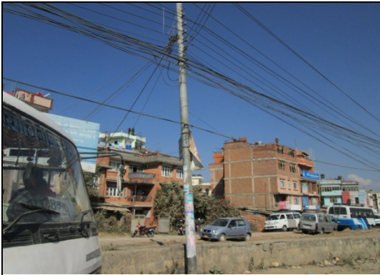
Figure 18. Electric poles no. 4
