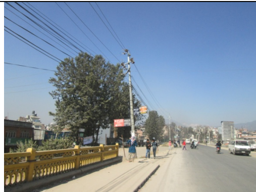
Figure 84. Electric pole no. 82
