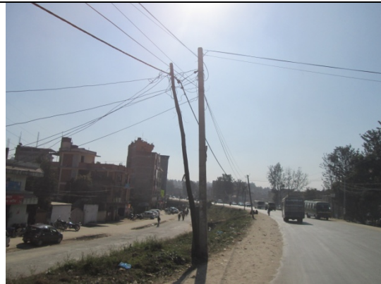
Figure 54. Electric pole no. 42 & 43
