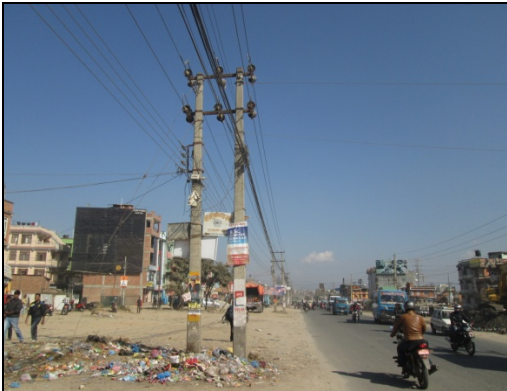
Figure 18. Electric poles no. 3
