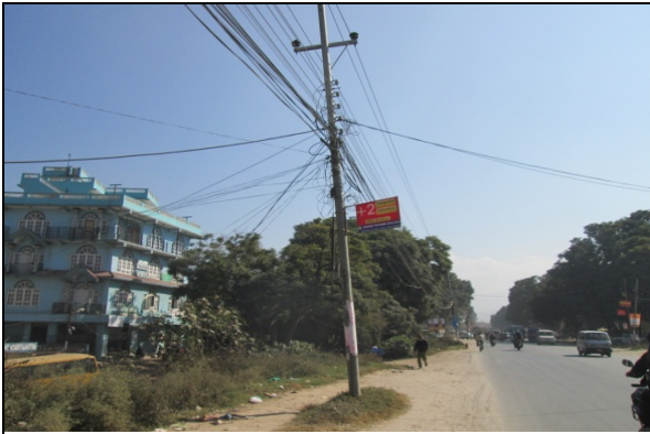
Figure 51. Electric pole no. 27
