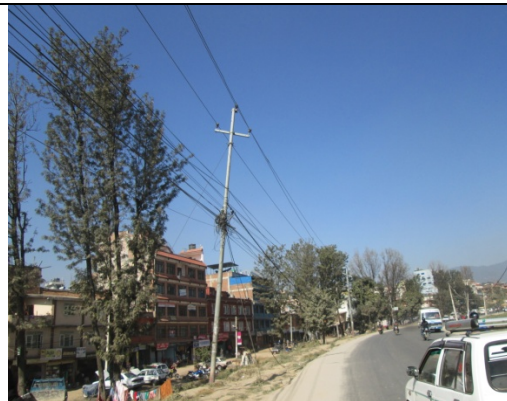
Figure 88. Electric pole no. 86
