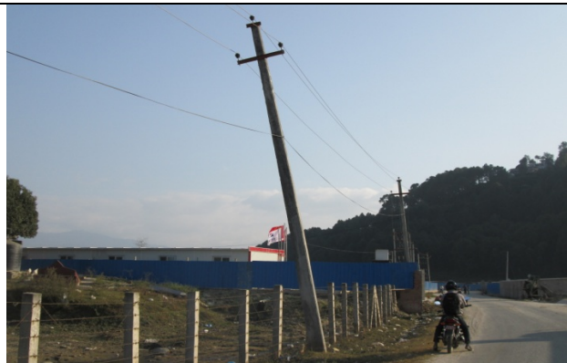
Figure 13. Electric pole no. 18
