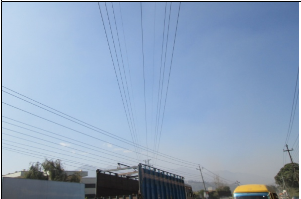
Figure 8. Crossing over of transmission line
