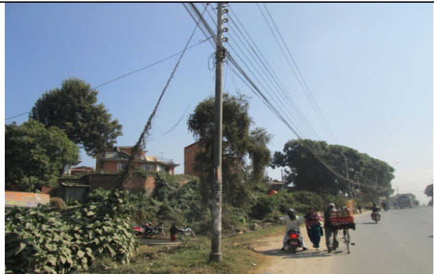
Figure 40. Electric pole no. 16
