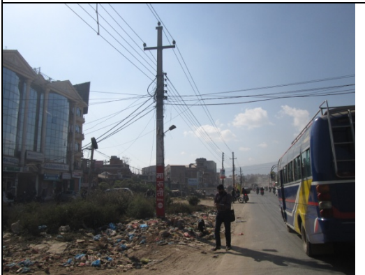
Figure 58. Electric pole no. 44
