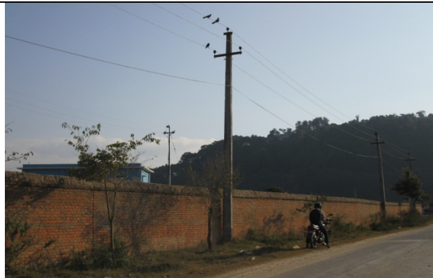
Figure 9. Electric pole no. 14
