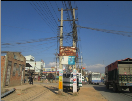
Figure 40. Electric poles no. 30
