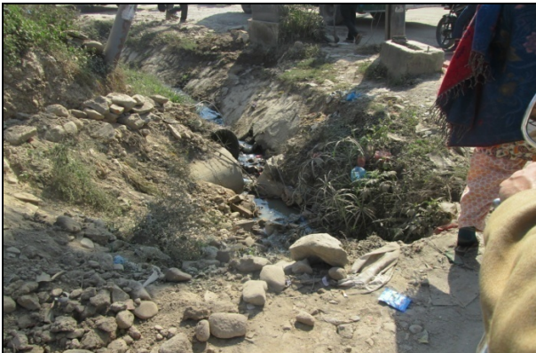
Figure 50. Underground sewerage and storm water drain
