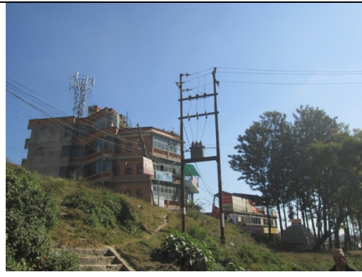
Figure 40. Electric pole no. 28
