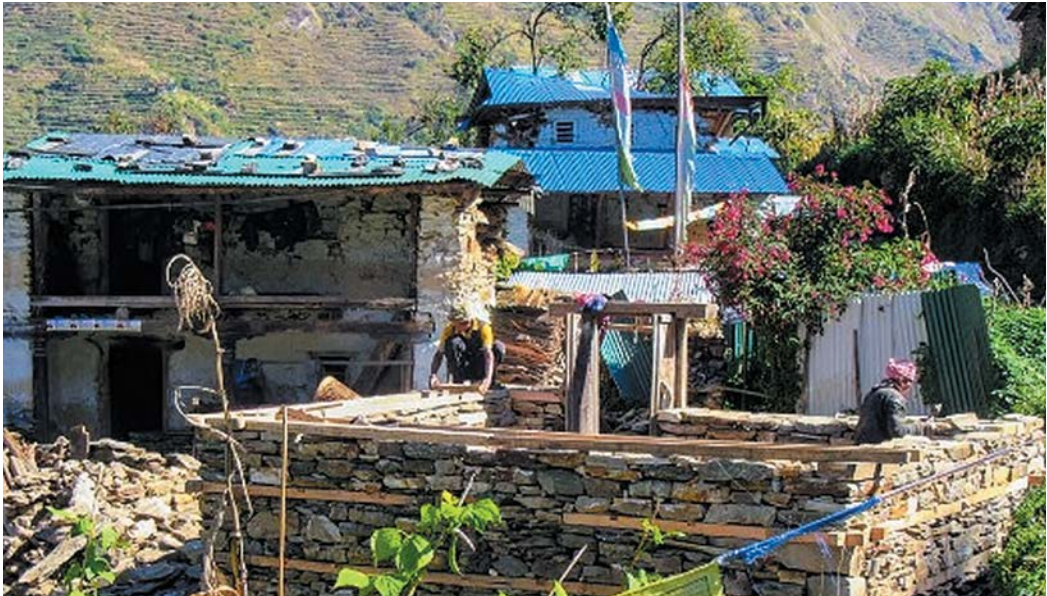
(A house under reconstruction in Tipling village, Dhading (Photo credit: Baliyo Ghar/NSET))
