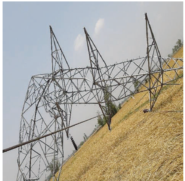
Full View of Collapsed Tower
