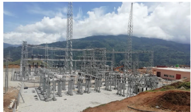
132/33/11 kV Tingla Substation
