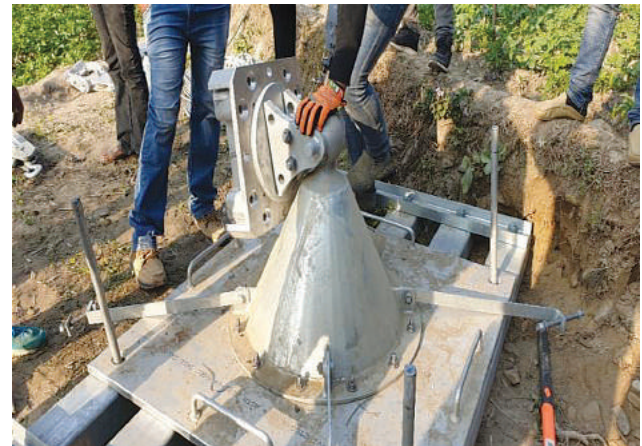
Foundation Setting Work for ERS Tower transmission line for Upper Trishuli 3A Hydroelectric Power Project can be constructed without long power
