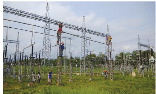
New Bharatpur Substation
