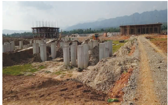
Construction of Control Building, Staff Quarter Building & Switchyard foundation is on progress
