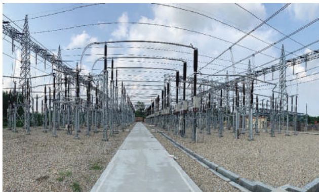
220 kV Substation at Dhalkebar
