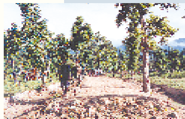
FfW road construction activities in the Terai are technically less demanding, but the labour management is very demanding.
