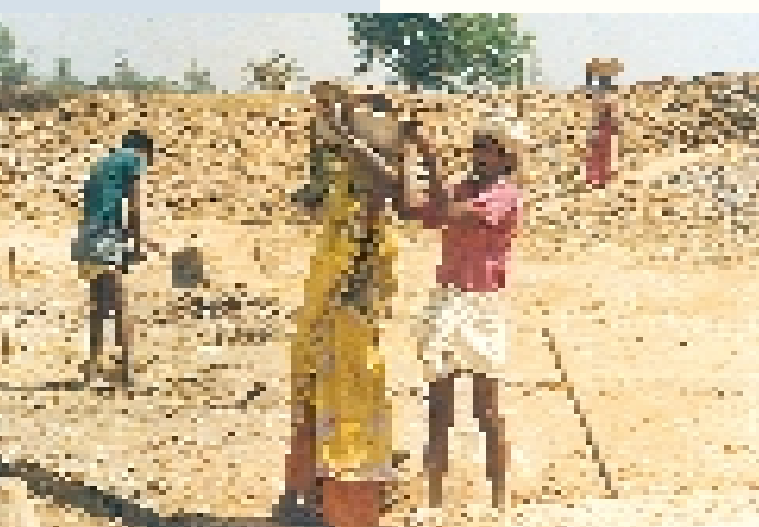
A typical Terai target group engaged in construction of a fish pond.
