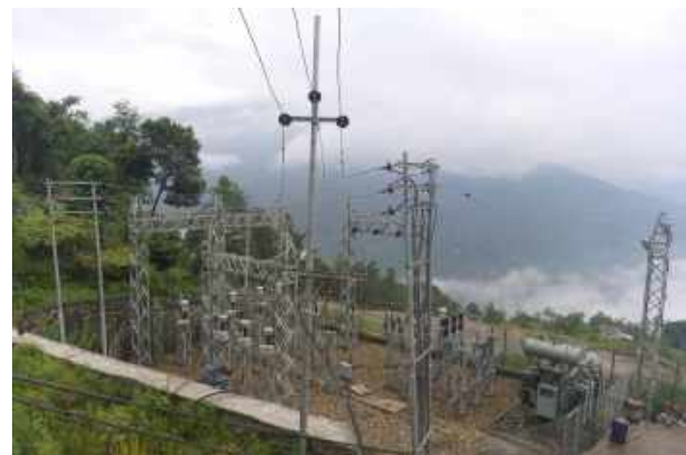
Photo: 33/11 kV, 6/8 MVA Substation at Taplejung
