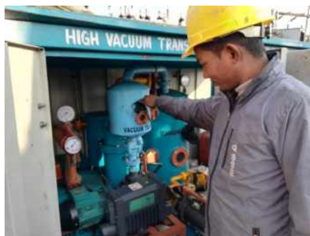
Oil Filtration for installation of 33/11 kV, 20/24 Power Transformer at Rani S/S, Biratnagar
