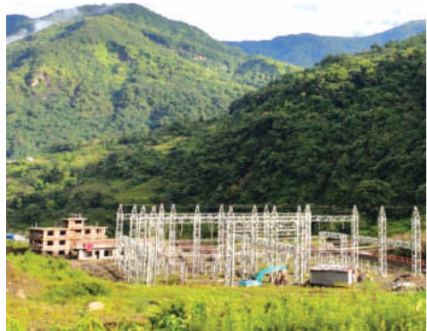
Kirtipur 132 kV substation
