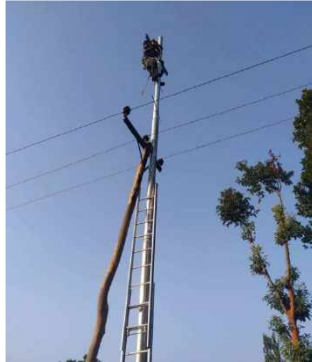
Replacement of non-standard and damaged wooden poles from 11 kV Line within Panchkhal DCS
