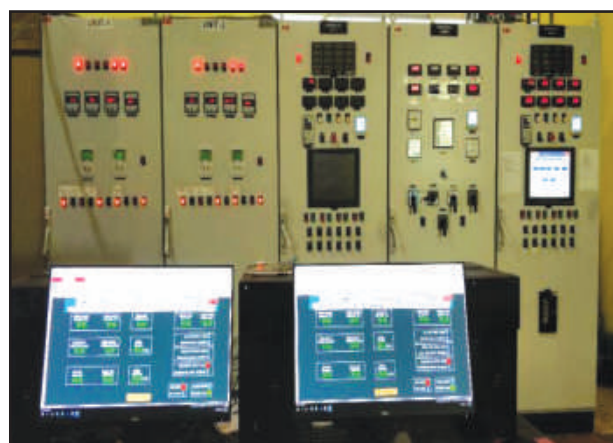
New Control Room
