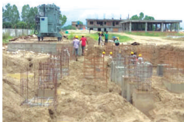
Nawalpur 132 kV SS
