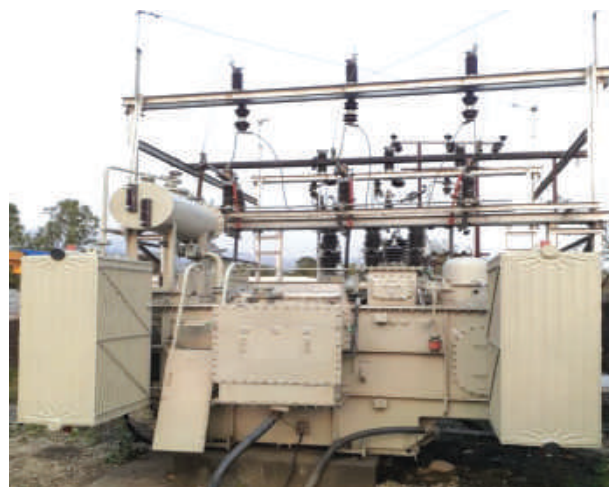
Power Transformer in the Switchyard
