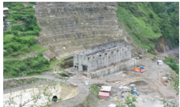
SUHEP Headworks & Powerhouse
