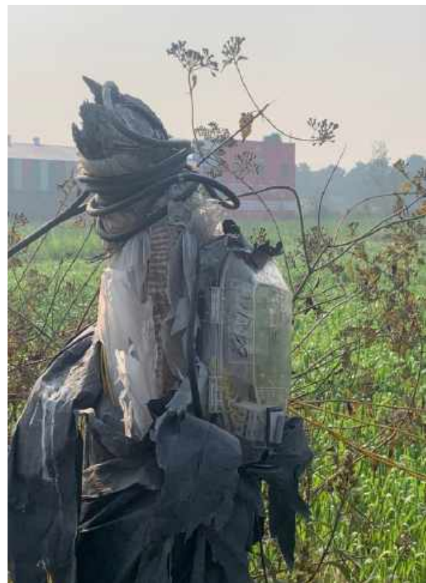
Irrigation meter hanged on a wooden local pole in Lahan DCS
