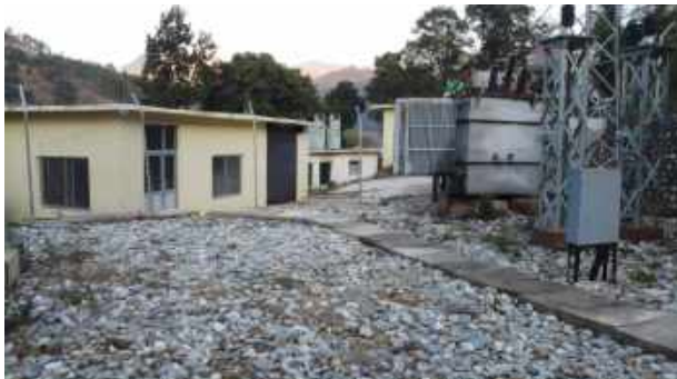
33/11 kV, 3 MVA Jhakale Substation at Achham
