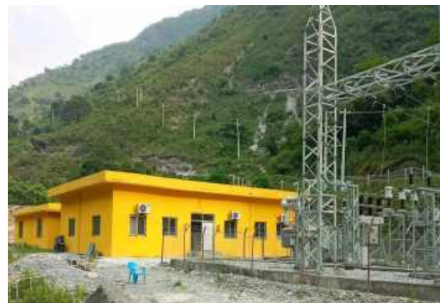
33/11 kV, 3 MVA Substation at Thaligaadh, Darchula
