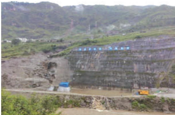
Under construction powerhouse filled with the water and debris during the flood.
