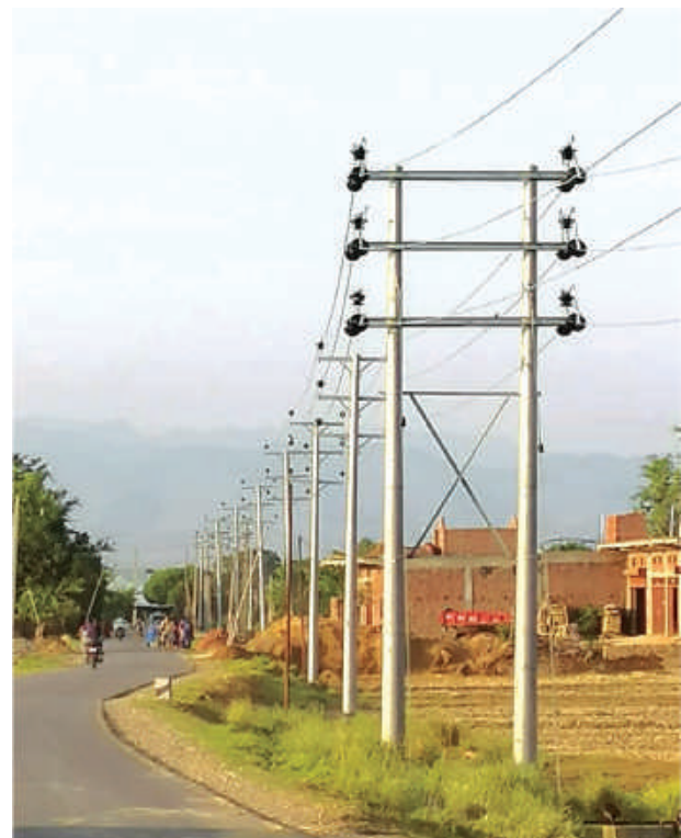
Butwal-Dhakdahi 33 kV line
