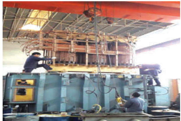
Tanking Power Transformer
