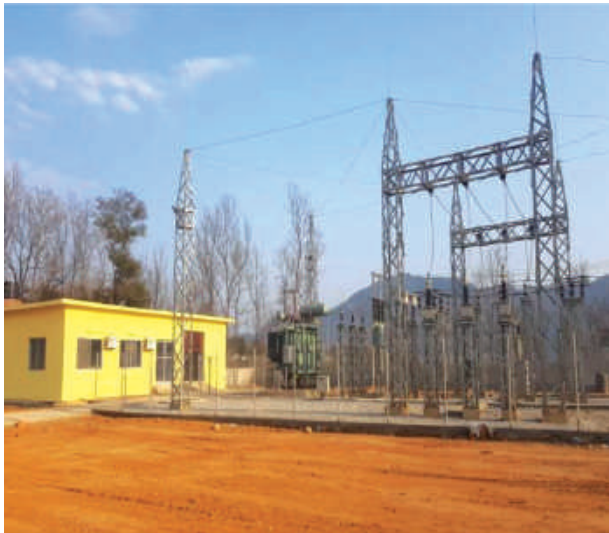
Khairenitar 33/11 kV Substation
