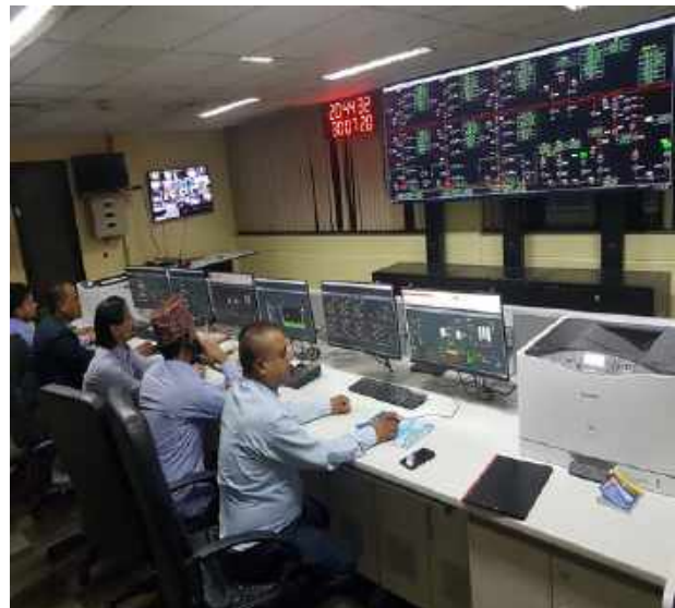
Control Room Furnished with SCADA
