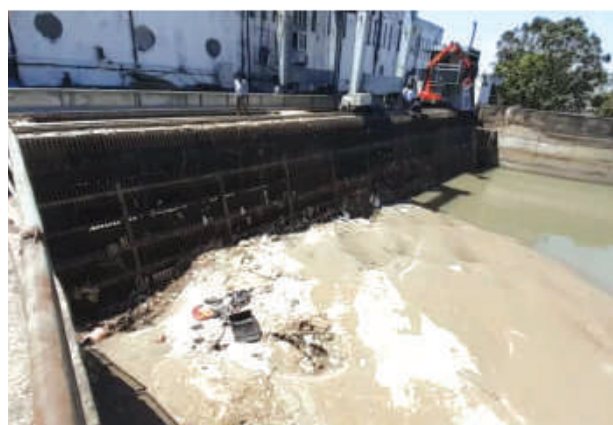
High sand deposition at Intake
