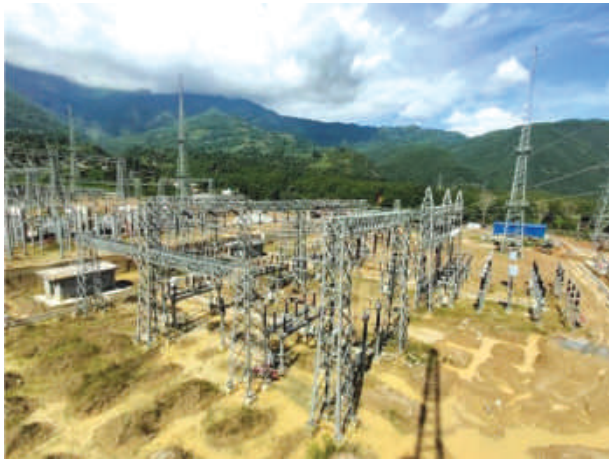
220 kV Kushma Substation
