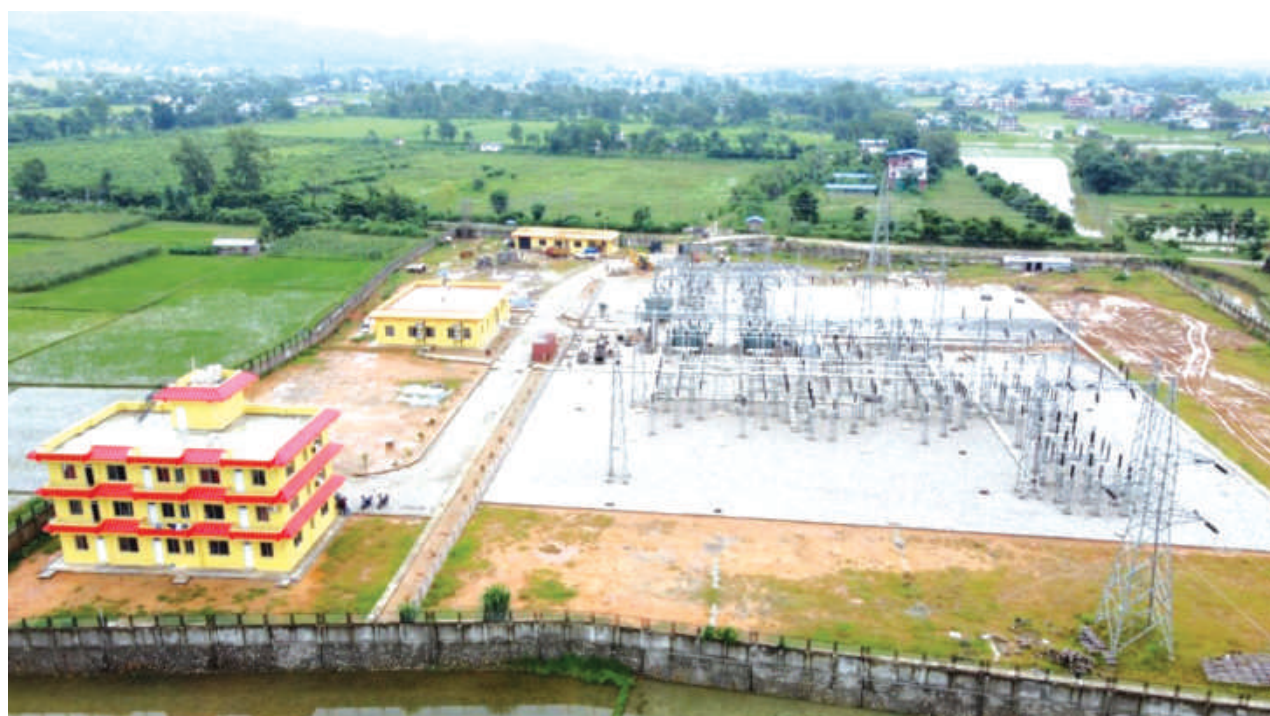
Purbi Chitwan 132 kV substation
