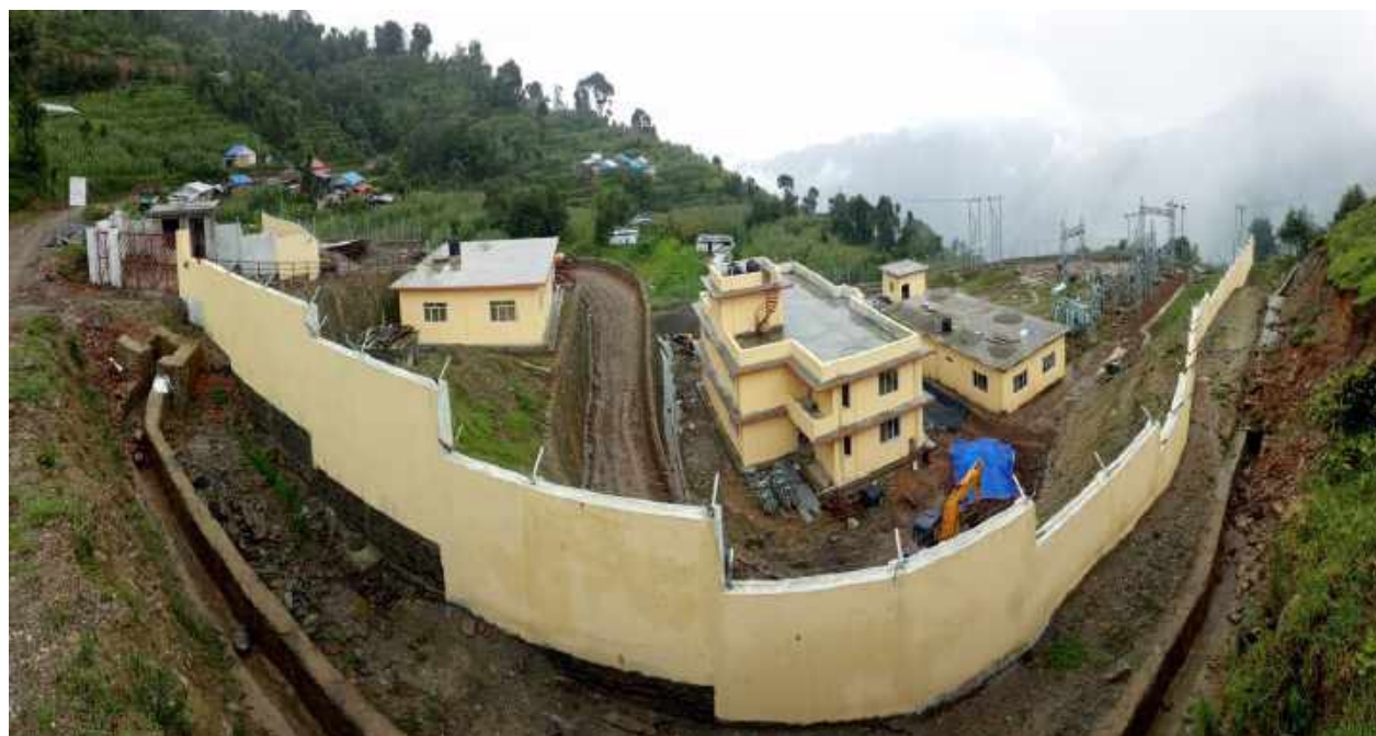
Panoramic view of 33/11 kV, 6/8 MVA Bhalche Substation, Rasuwa
