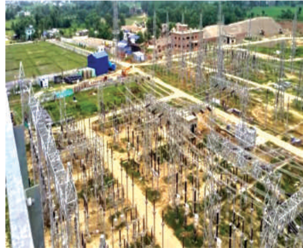
Switchyard of 220 kV New Butwal Substation
