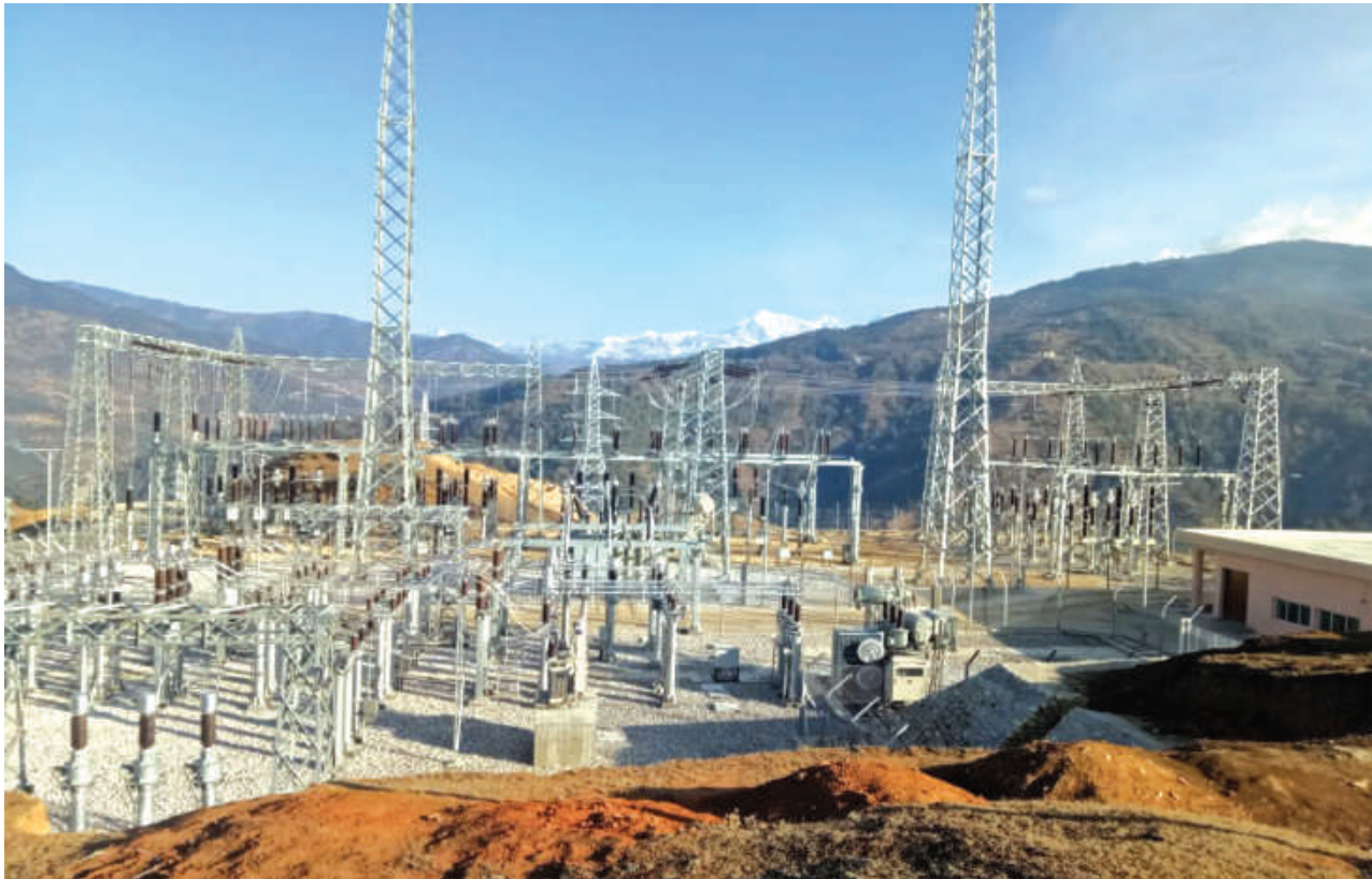
132/33/11 kV Tingla Substation
