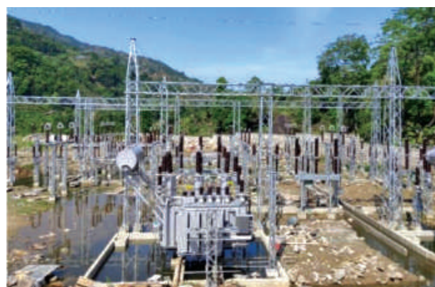
Samundratar 132/33 kV Substation
