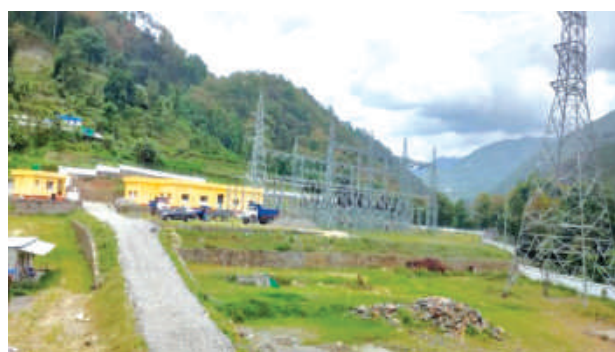
New Modi substation
