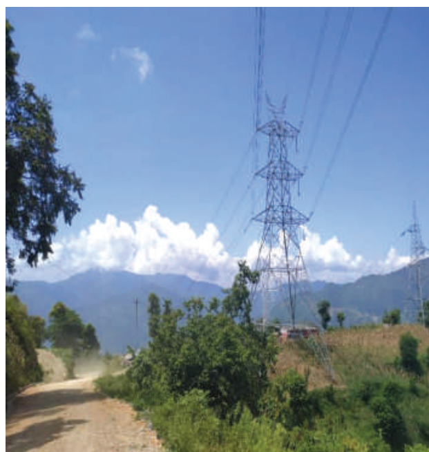
Marsyangdi- Kathmandu 220 kV Transmission Line
