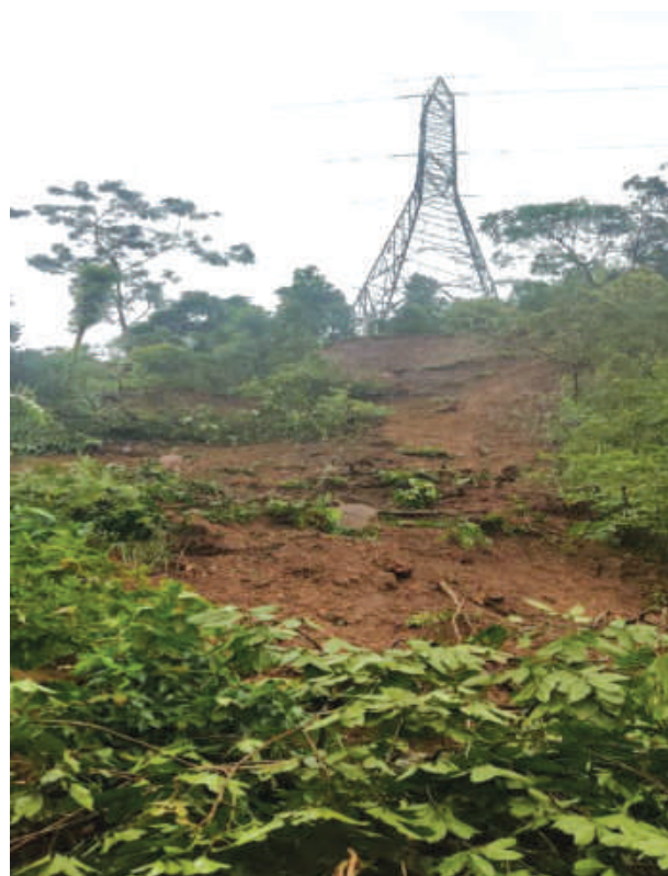
Landslide near Tower no.31 in Kaligandaki Syangja 132 kV section
