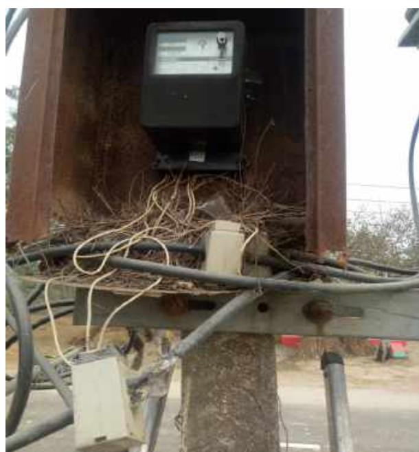
CT operated electromechanical meter found in Janakpur DCS (PT outage )
