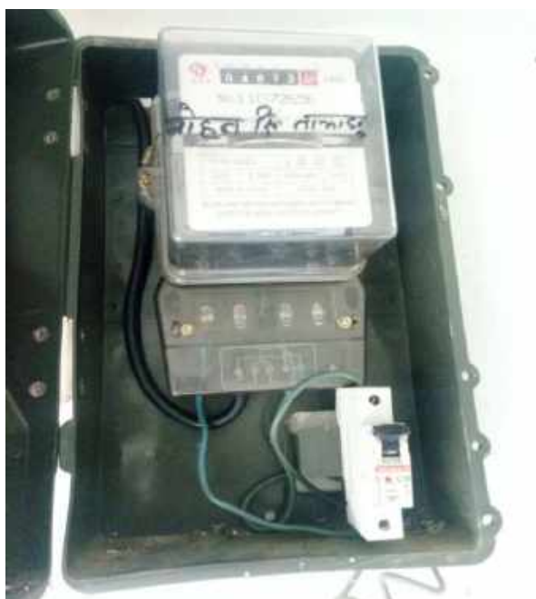
Single phase meter bypass found in Kabhre DCS
