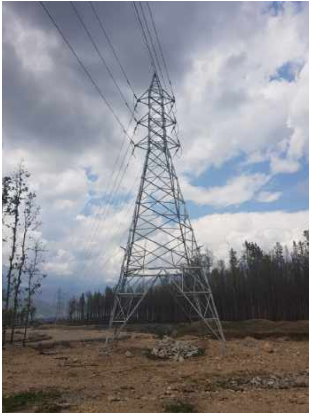
Tower Erection for 33 kV Line from Kamane to Riddhi Siddhi Cement Industry
