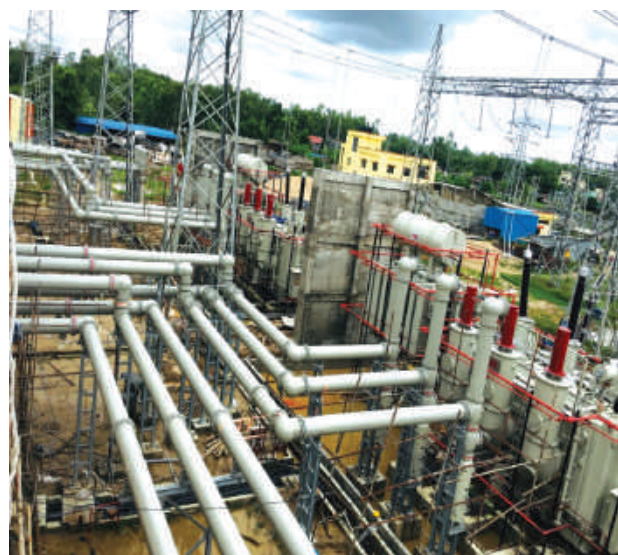
400 kV GIS Hall at Dhalkebar 400 kV Transformer at Dhalkebar
