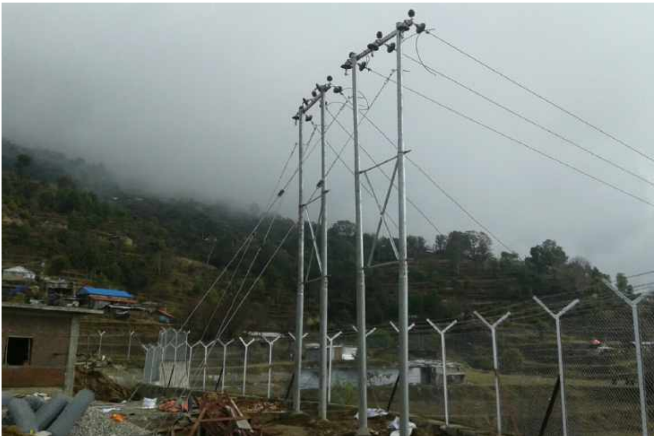
11 kV outgoing feeder from Bhalche Substation to neighborhood areas
