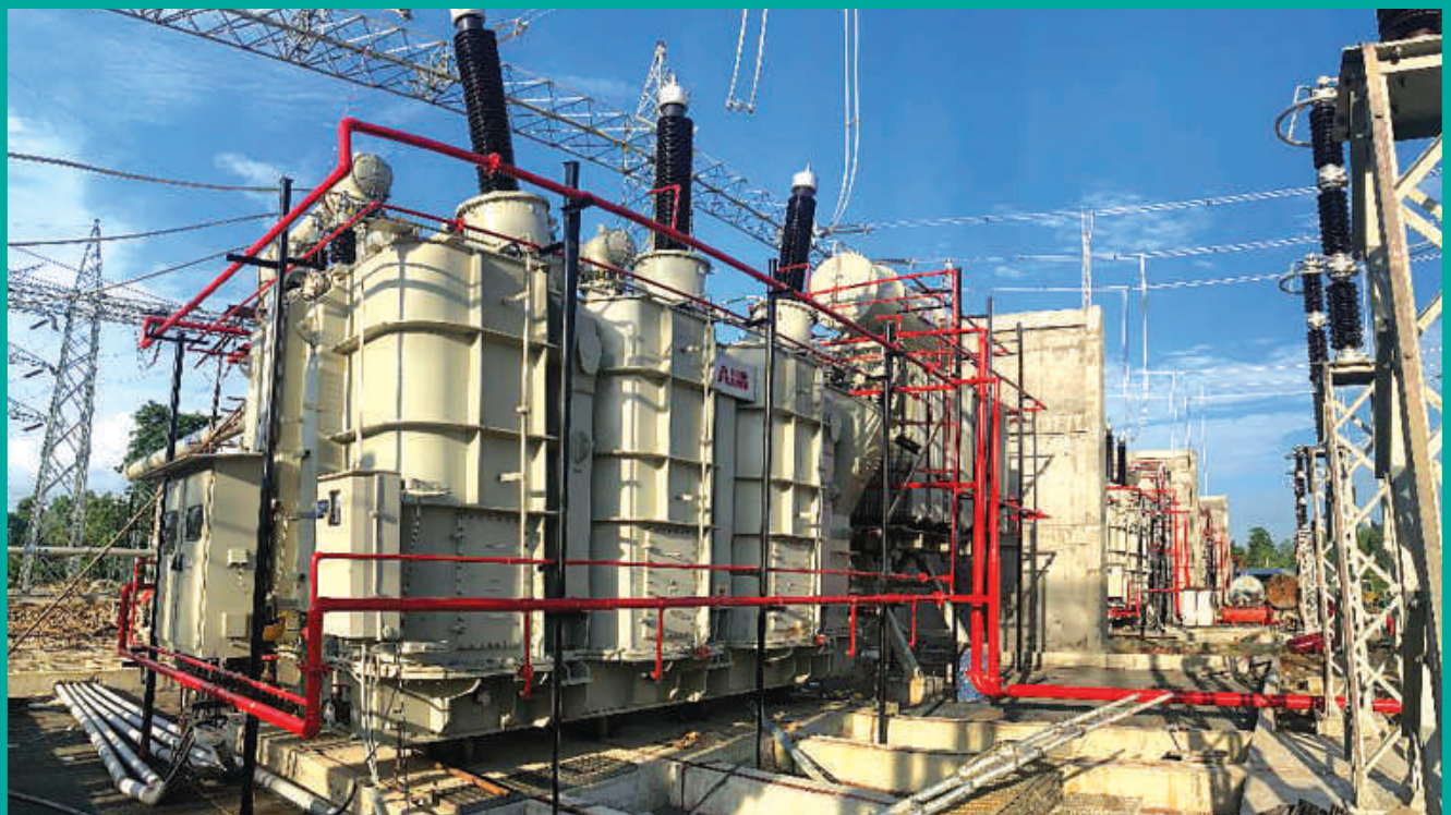
Dhalkebar 400/220 kV Substation
