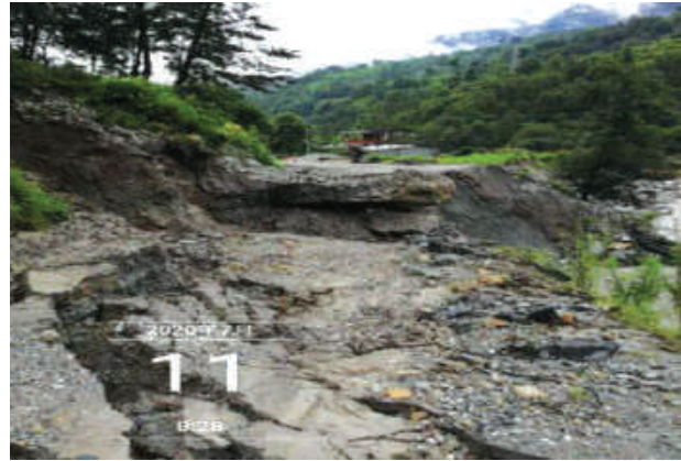
Severe damages observed in Araniko Highway (Access to the Project Site) during the flood.
