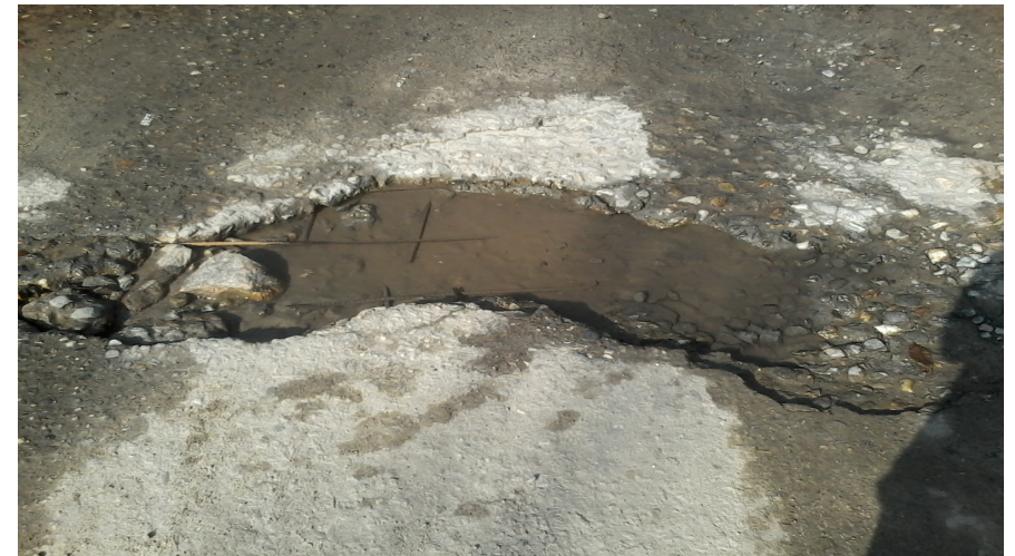
Caption:crack and rebar exposed in running surface
