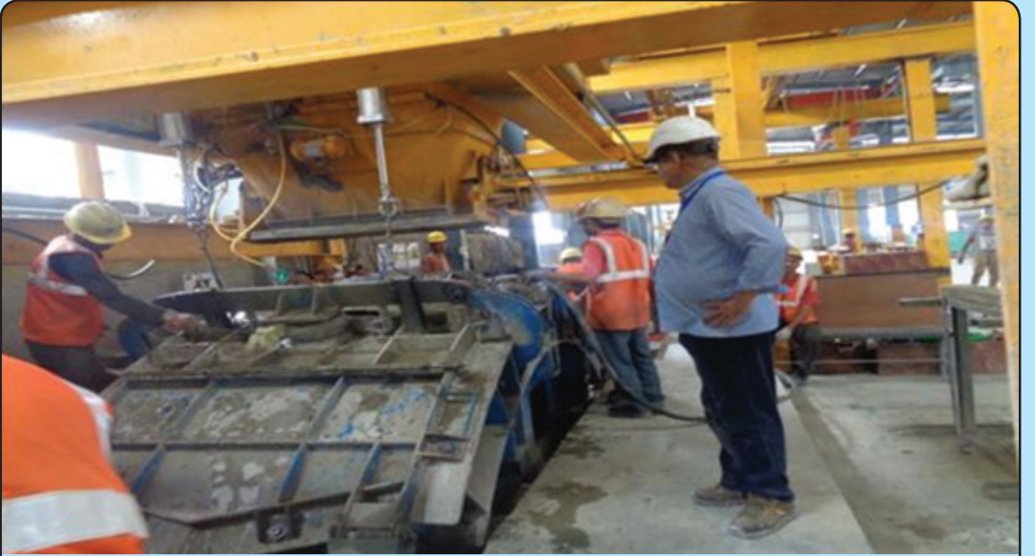
Inspection of quality of concrete, Bheri Babai Diversion Multipurpose Project, Birendranagar, Surkhet
