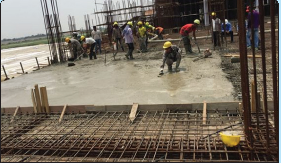
RCC slab working at ITB, South Asia Tourism Infrastructure Development Project, Gautam Buddha Airport, Rupandehi, ICB 01 Construction of Airside and Landslide Infrastructure and other Facilities
