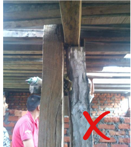
Two post are not connected.
